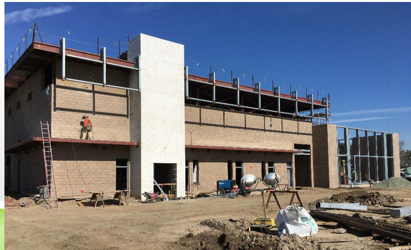
New Central Plant
